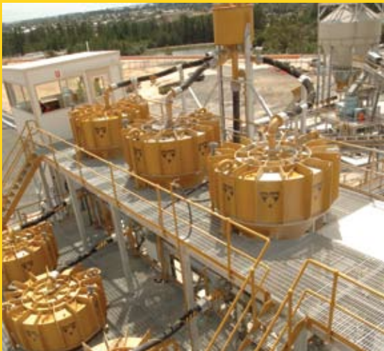
BGF gravity plant - designed and installed by Gekko.
